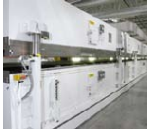
Dryers and Ovens
