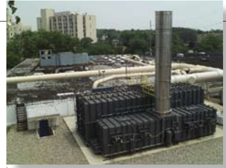
Exhaust from a flexible packaging plant is purified by an Enterprise II regenerative thermal oxidizer
