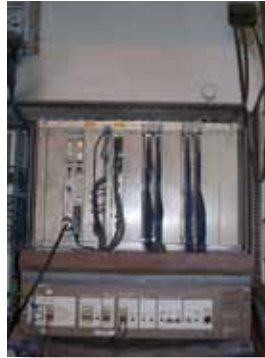
Old S5 Siemens S5 PLC
