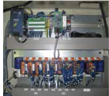
SAIA PLC Upgrade
