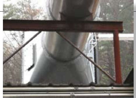
Process Heating Coil
